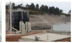
Odor collection and treatment in environmental protection zone
