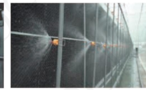
Spray deodorization at rear end of fan
