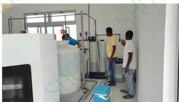
A water plant in Zambia
