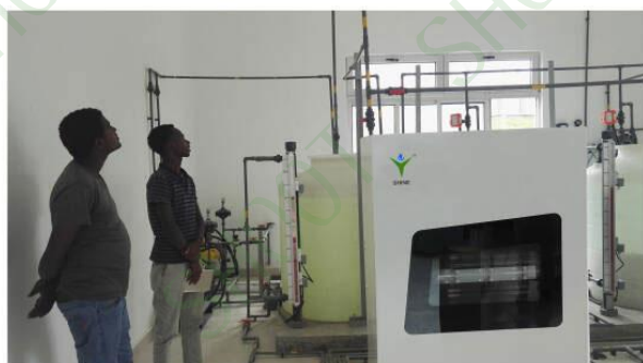
A water plant in Zimbabwe
