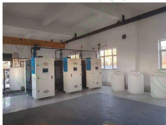
A sewage plant in Jiangxi, China
