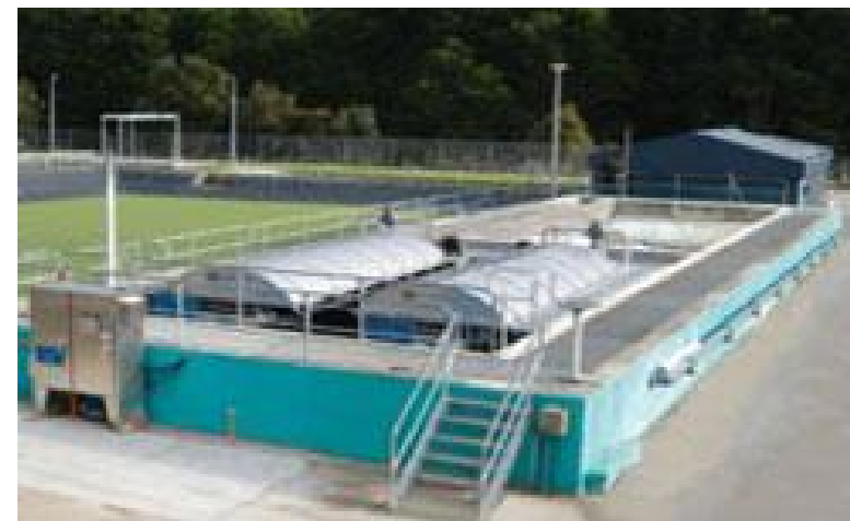
Water treatment plant
